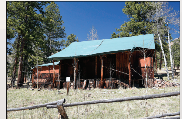
Thanks to funding from the Friends of Staunton State Park, tarps were installed over the cabin roof in May 2020 to slow further deterioration to the Staunton Homestead Cabin.
