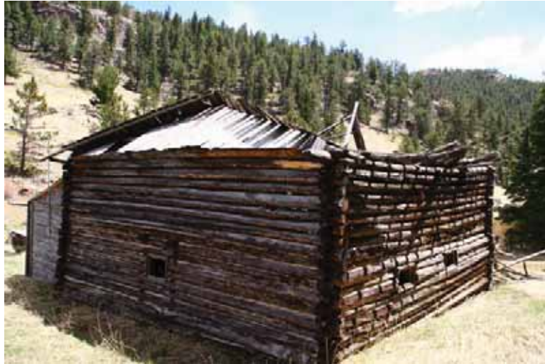
Figure 7: Exterior View of Collapsed Barn
