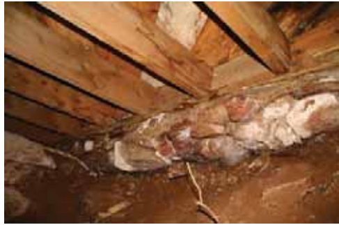
Figure 28: Undercut Foundation in Cellar
