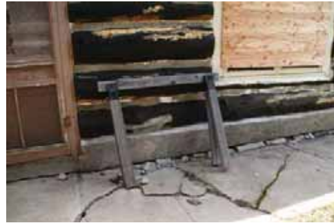
Figure 26: Foundation and Damaged Sidewalk
